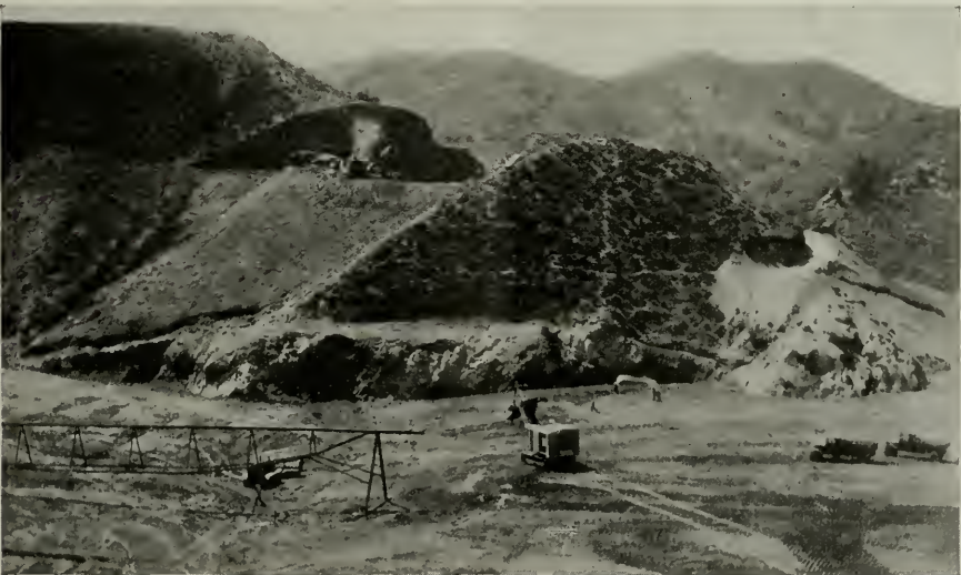
Spillway is excavated in shale of west abutment. Shovels strip valley fill to bedrock in upstream portion of dam.
